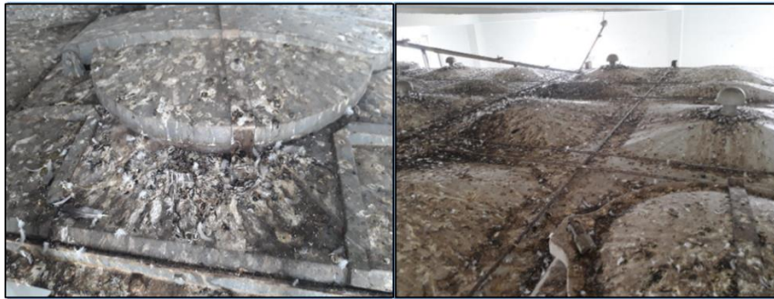
Presence of bird droppings on water tanks
