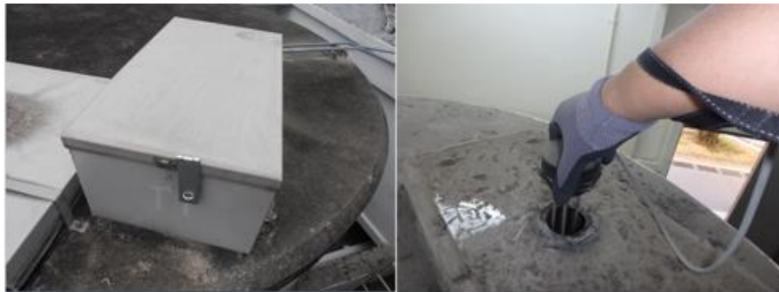
Electrode box cover and holder not properly secured
